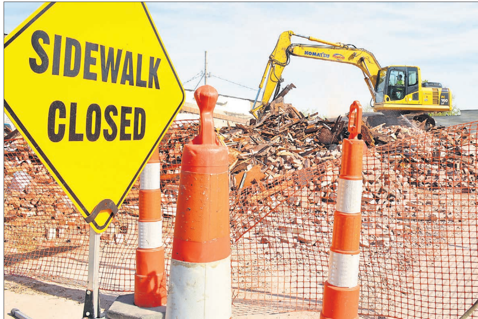
Steven Pleasant Excavating employee Adam France works Monday to remove scrap materials from the former Givens Book Exchange site in Madisonville. A total of 14 dump truckloads of used books were removed from the condemned store prior to its demolition on Sunday.
