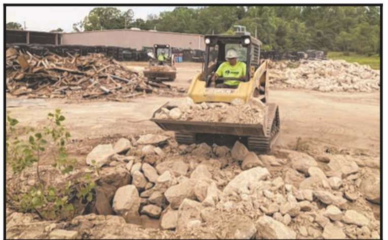
Workers from Alliance Service Group of Grove City, Ohio, use skid loaders Wednesday to fill pits in the yard at the former Dana Corporation foundry site. BILL ENGLE/PALLADIUM-ITEM
