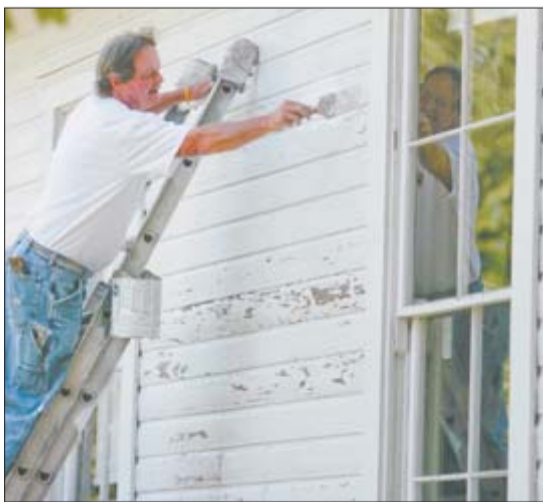
ROBERT K. YOSAY | THE VINDICATOR Ray Blair of Jewels Airless Spray Painting of Hubbard paints the schoolhouse in Western Reserve Village at the Canfield Fair. The work is part of $174,700 in improvements to this year's fair, which starts Wednesday.
